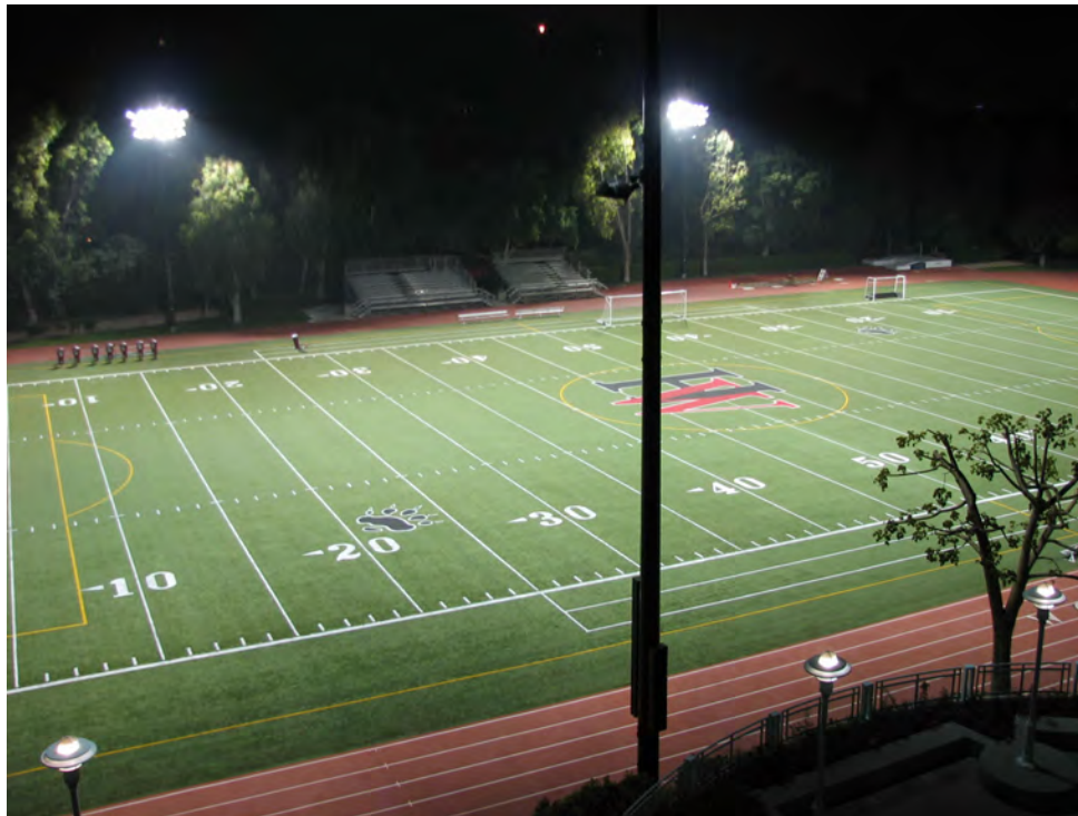
Figure 3.1-28 Night Lighting of Ted Slavin Field and Track Illustrating Precise Targeting of Lighting and Limited Spillover Lighting
